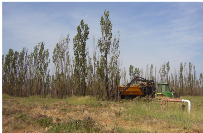
Rehabilitation of the site: removing old orchard and windbreaks, irrigation equipment and other agricultural residue
